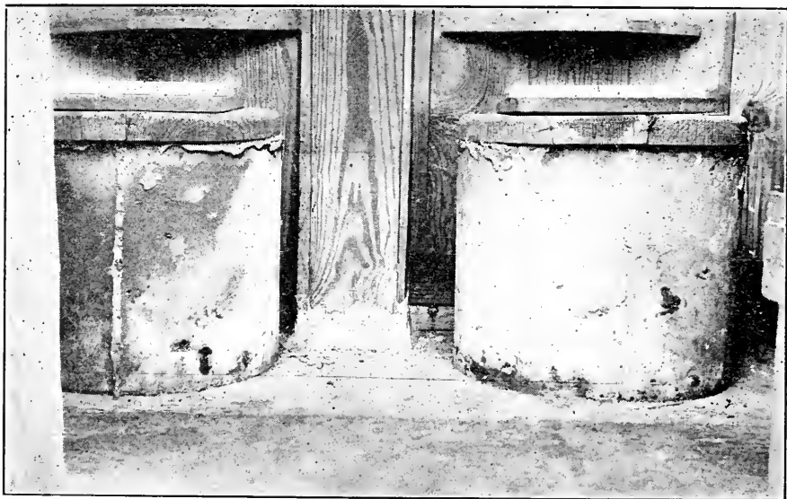
FIG. 6. Excellent seats, but faulty seat covers. Always be on guard for warping such as seen in this picture. This furnishes ample opportunity for flies to reach the privy contents.
