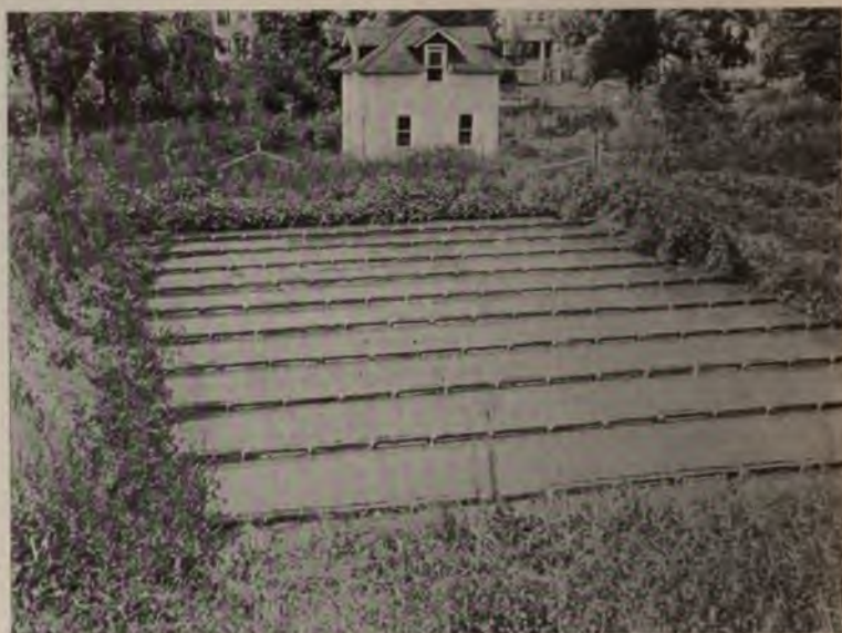
Fig. 48.—The distributing troughs on the sand filter of a small sewage disposal plant.
