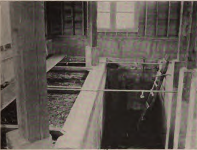
Fig. 43.—Two settling tanks—one empty and one filled.
