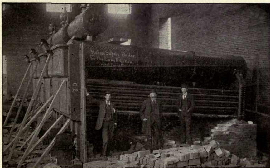
Boiler Plant of Lannett Cotton Mills, WEST POINT, GA. 900 H. P. Heine Boilers.
