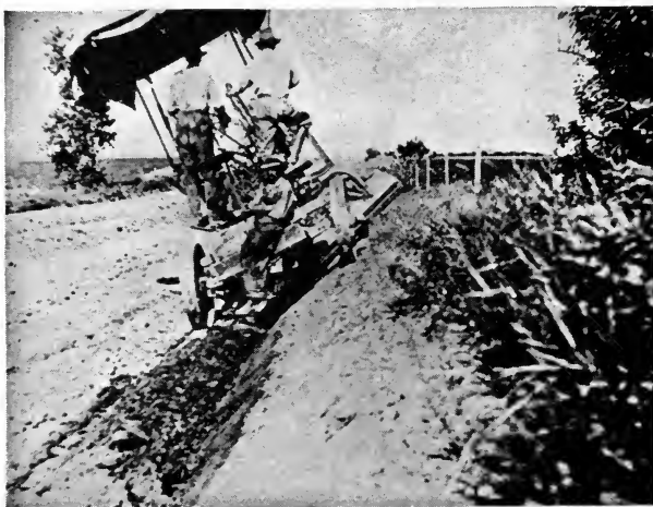
FIG. 77.—Trimming Off the Side with a Road Grader on a State-aid Project in Nebraska.
