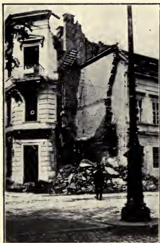
This was formerly a drug-store in the center of Belgrade. A large 42-centimeter shell passed entirely through the three stories down into the basement and exploded, completely demolishing the entire building, killing instantly several of its occupants and shattering windows for squares in the vicinity.
