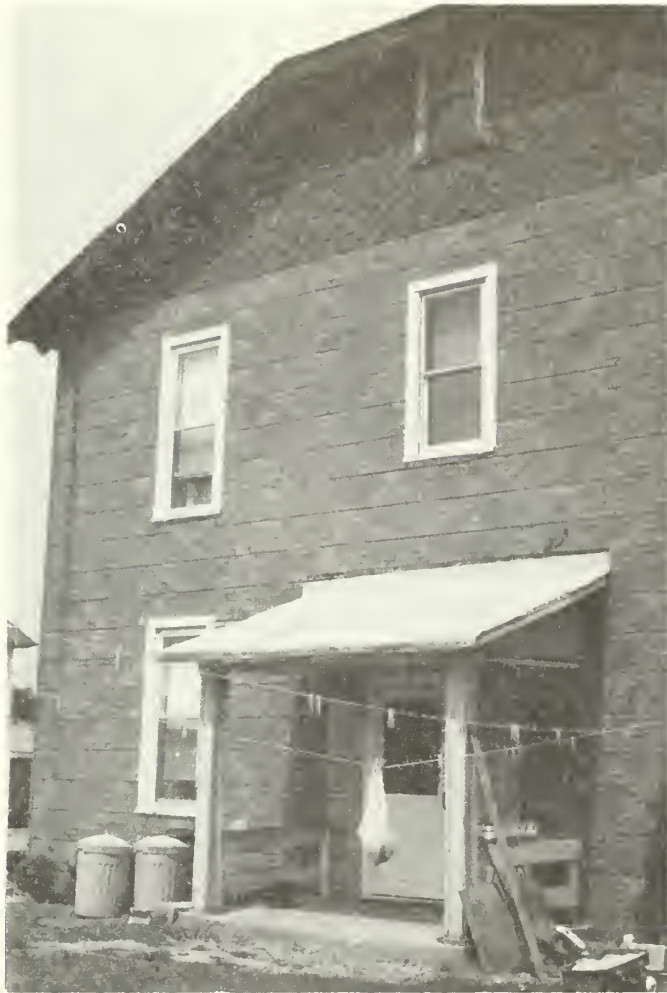
Photo E-96 Detail of west elevation showing original wood siding flanking rear door. Clubhouse Annex 1992
