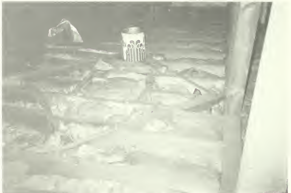
Photo E-31a View of third floor ceiling framing from attic showing framing for ventilator. Clubhouse 1992
