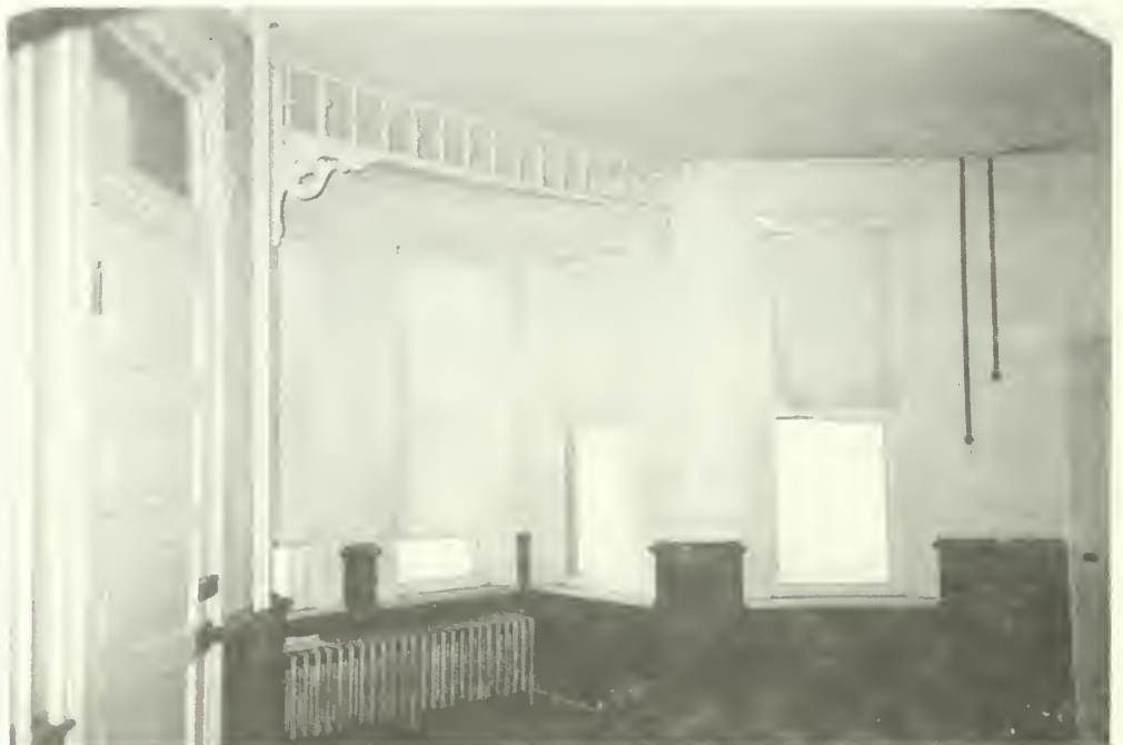
Photo E-42 Northeast bay with decorative wood bracket in room 106. Brown Cottage 1992
