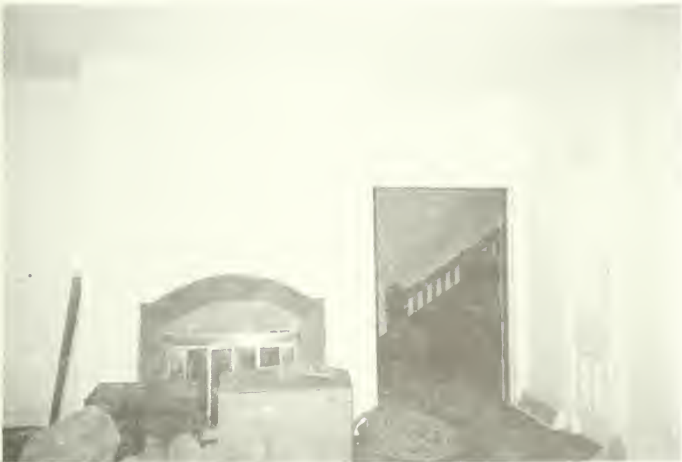
t) E-77 South wall and fireplace of room 104 with view of main stair to the right. Moorhead Cottage 1992
