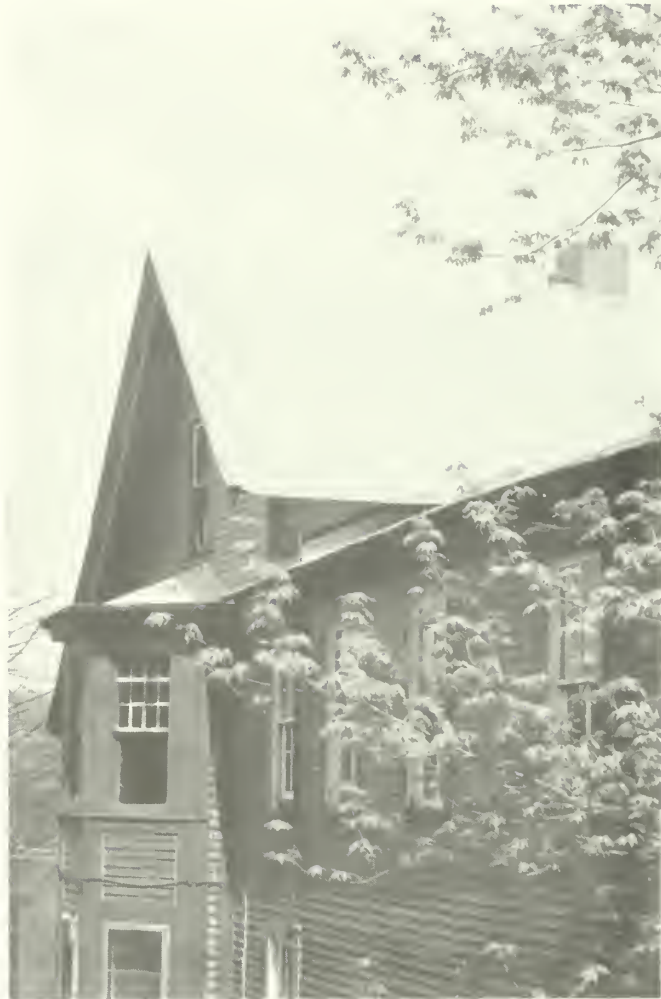
Photo E-64 North facade showing original wood shiplap siding visible at the eave of the main roof and in the return of the bay area. Moorhead Cottage 1992
