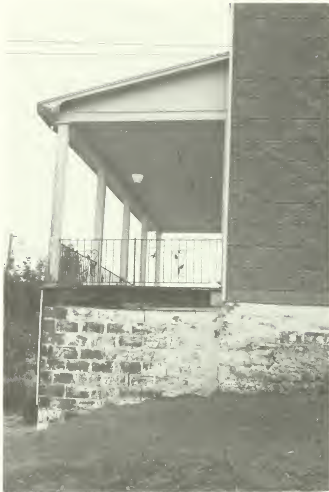
Photo E-97 Detail of the north foundation wall showing original stone foundation with brick and concrete block infill above. Clubhouse Annex 1992
