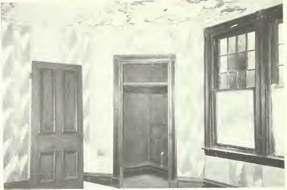
Photo E-84 Northeast corner of room 202, showing original door, as well as door and window casing with rose blocks. Moorhead Cottage 1992
