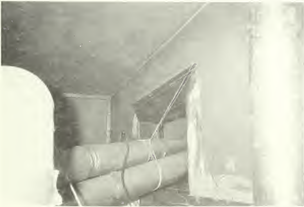
E-18 View above existing kitchen ceiling of room 107, looking northeast at east wall of original center hall and door opening. Clubhouse 1992
