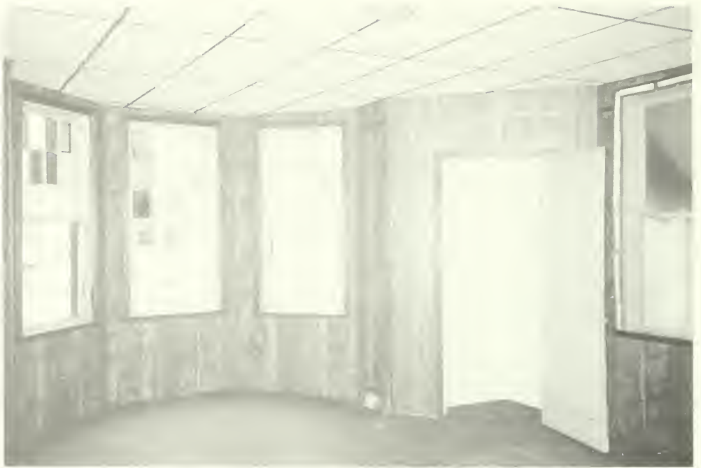
Photo E-88 North bay and northeast corner of room 204, showing colored glass in upper sashes of bay and modern paneling. Moorhead Cottage 1992
