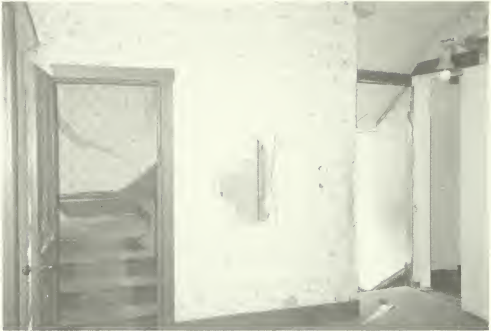
Photo E-81 View of enclosure added over main stair at second floor. Moorhead Cottage 1992
