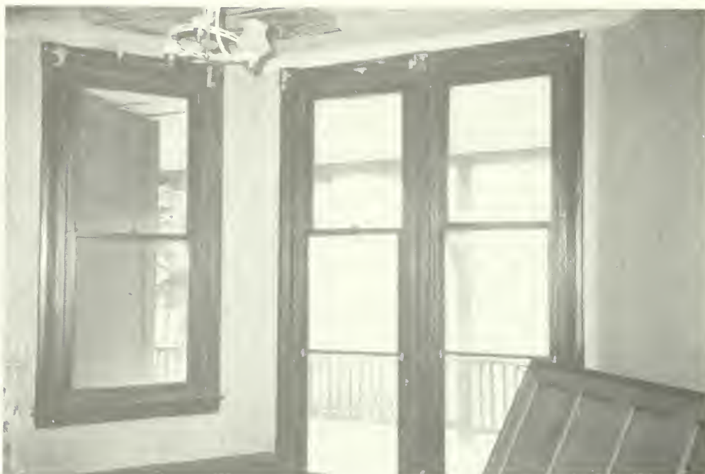
Photo E-74 Northeast and east walls of room 102, showing tall double hung windows opening onto porch. Moorhead Cottage 1992
