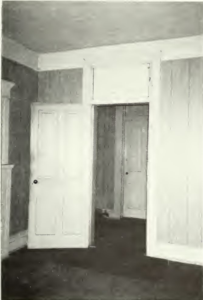
Photo E-27 Typical door and transom at second and third floor guest rooms. Clubhouse 1992
