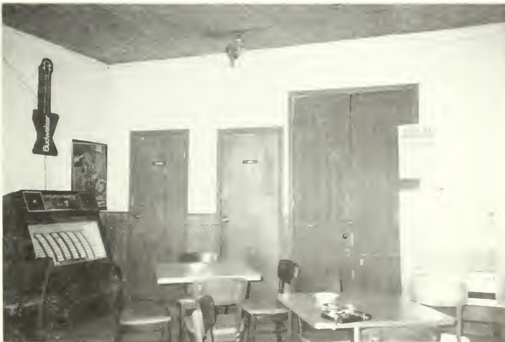
c E-15 West wall of room 102. Although the wall is new, the double doors are original and have been relocated. Clubhouse 1992
