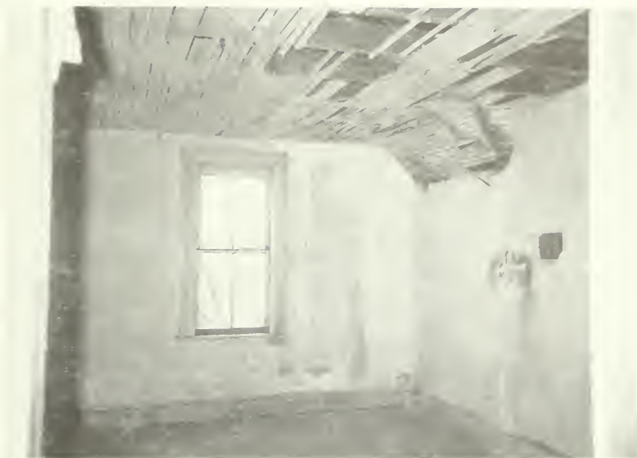
Photo E-90 Southeast corner of room 301, showing deteriorated wall and ceiling plaster. Moorhead Cottage 1992
