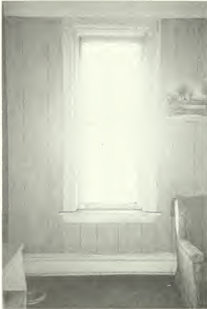
Photo E-26 Typical second and third floor baseboard and window trim. Clubhouse 1992
