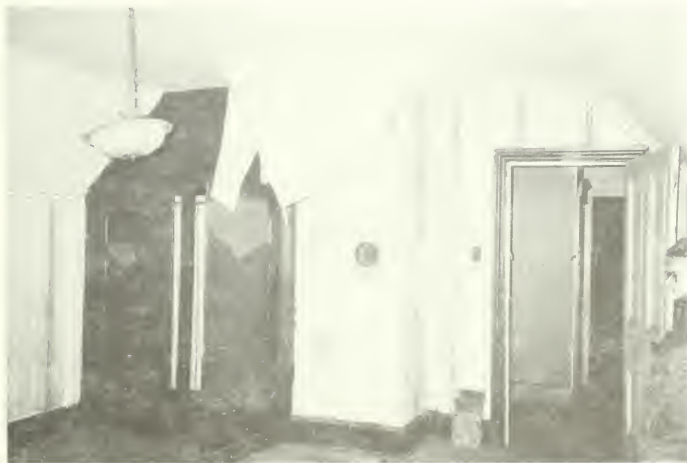
Photo E-91 South wall of room 304 with view to hall 300. Closet to the left is a later addition. Moorhead Cottage 1992
