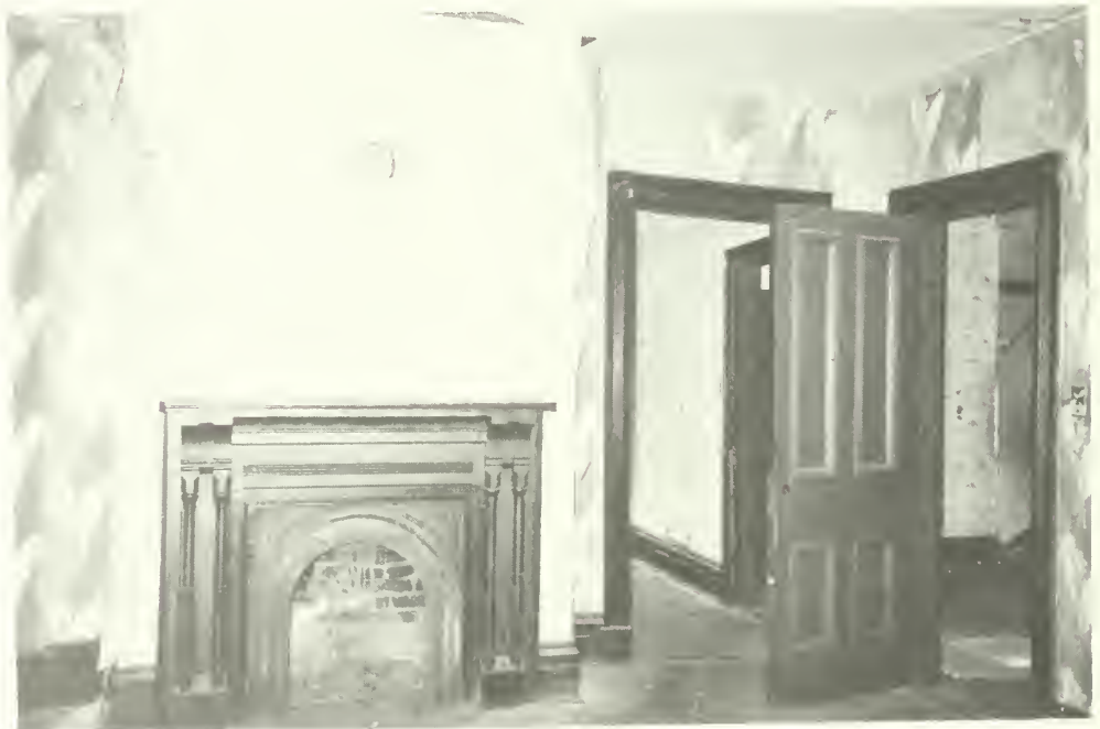
Photo E-85 Northwest corner of room 202, showing fireplace and mantel. Moorhead Cottage 1992
