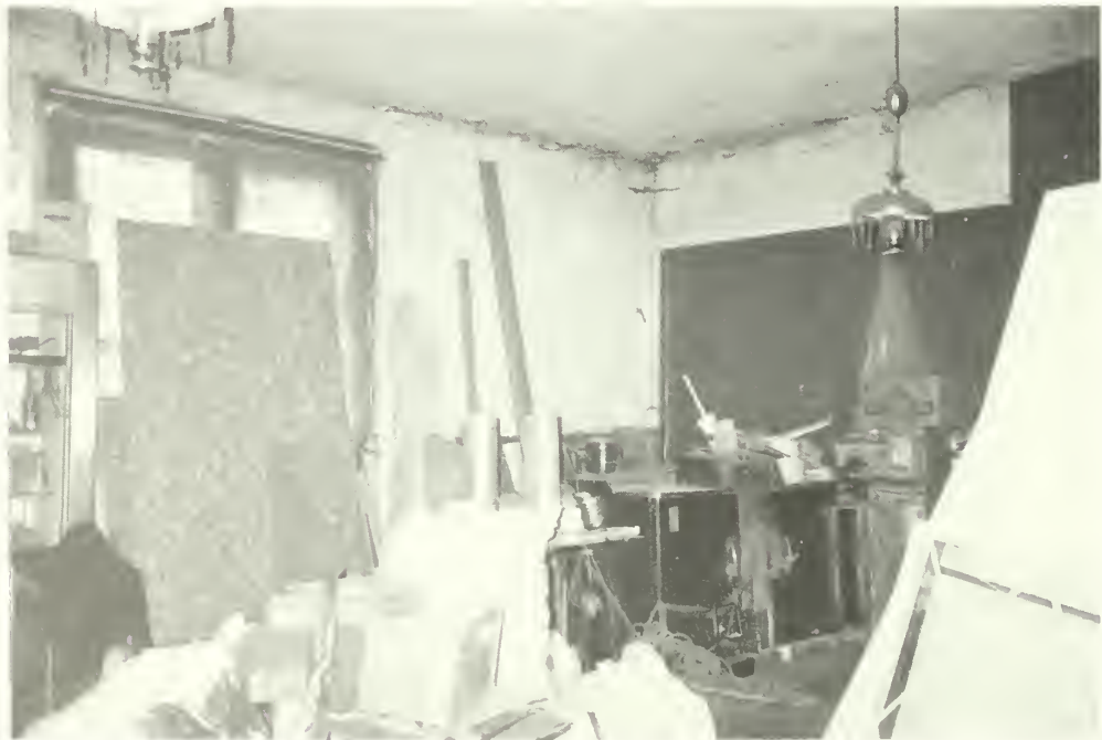
Photo E-20 Looking northwest in room 114 towards window in west wall and newer, large cased opening in north wall. Clubhouse 1992
