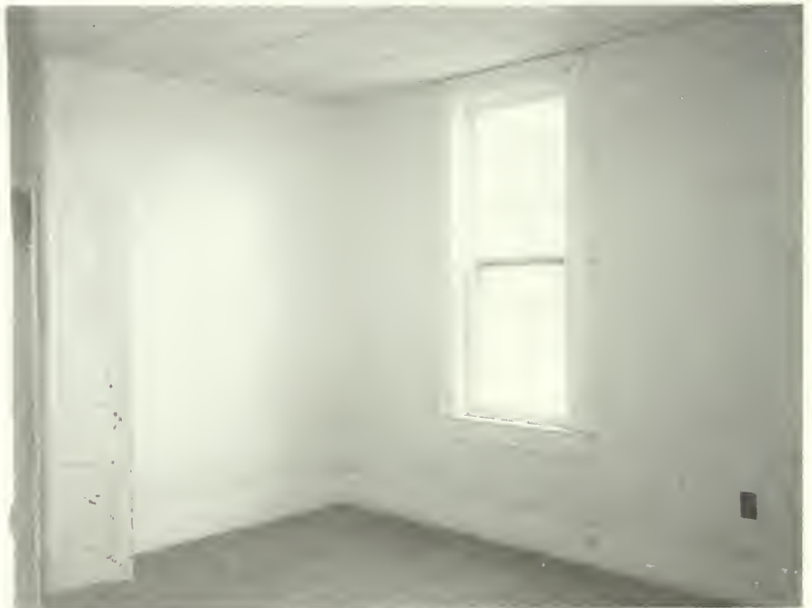
Photo E-52 Northwest corner of room 208. The door to the left leads to the newer stair to the third floor. Brown Cottage 1992
