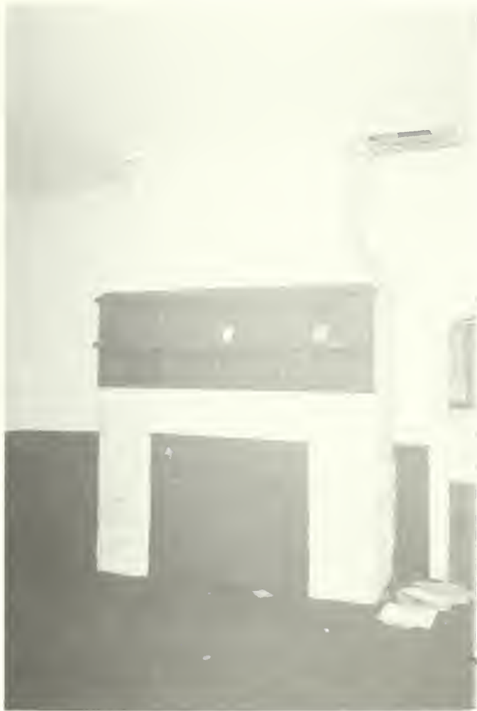
Photo E-43 Chimney and fireplace on west wall of room 106. Brown Cottage 1992
