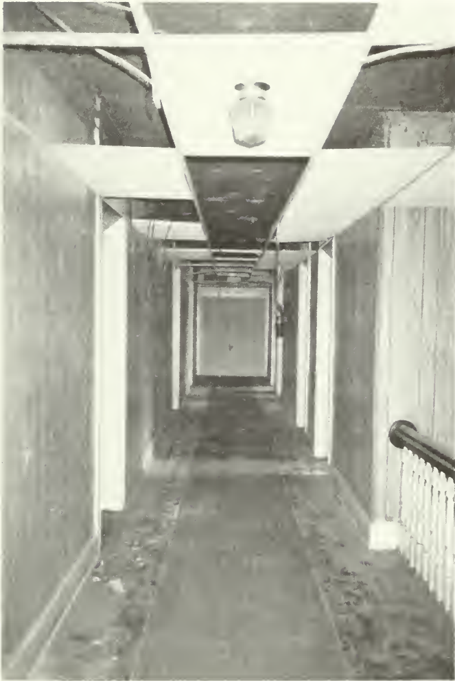
Photo E-25 Second floor hall, looking south. Note railing for main stair at right of photo. Clubhouse 1992
