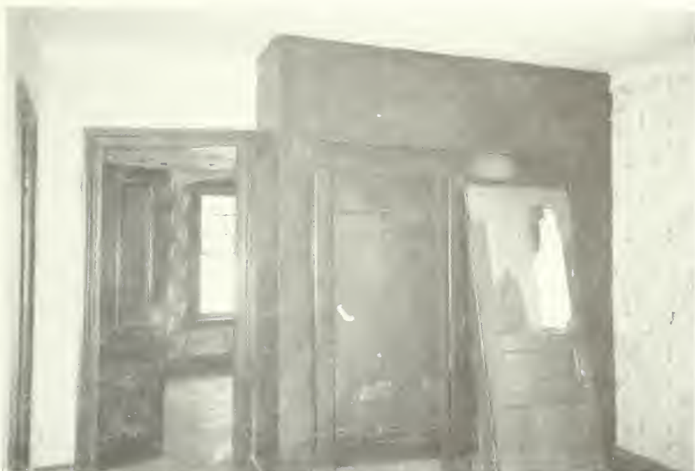
E-86 East wall of room 203 with view through doorway to room 202. The closet is an addition to the room. Moorhead Cottage 1992
