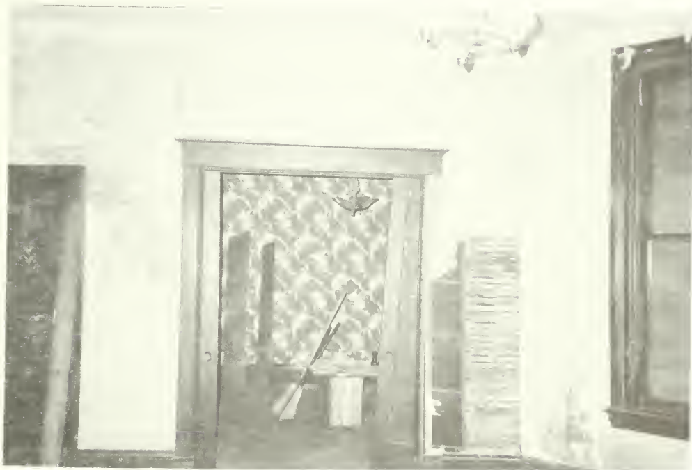
c E-73 North wall of room 102 showing early twentieth century pocket doors and alterations to wall. Moorhead Cottage 1992
