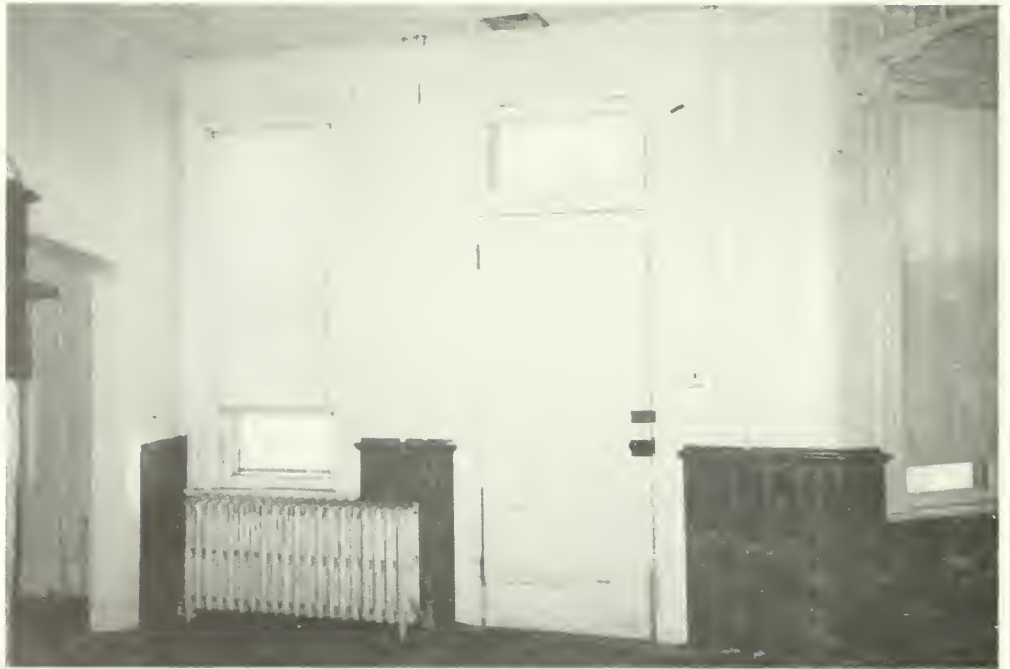
Photo E-41 North wall of room 106. Although the wood wainscot is original, the original entry door has been replaced. Brown Cottage 1992
