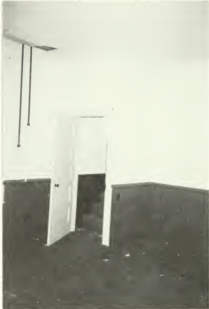
Photo E-44 Southeast corner of room 106 showing enclosed stair added during the Mining Company Era. Brown Cottage 1992
