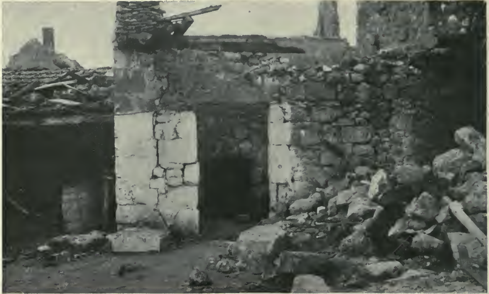
Deflated Entrance to Wine Cellar First Occupied as H Company P. C. in St. Thibaut.
