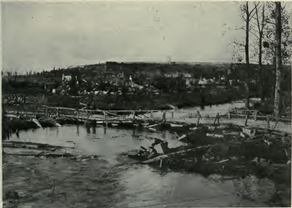
Bridge Hastily Constructed by 302nd Engineers over Vesle River between St. Thibaut and Bazoches.
