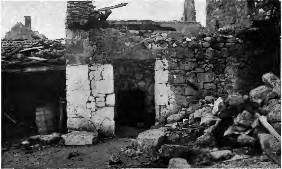
Defiled Entrance to Wine Cellar First Occupied as H Company P. C. in St. Thibaut.
