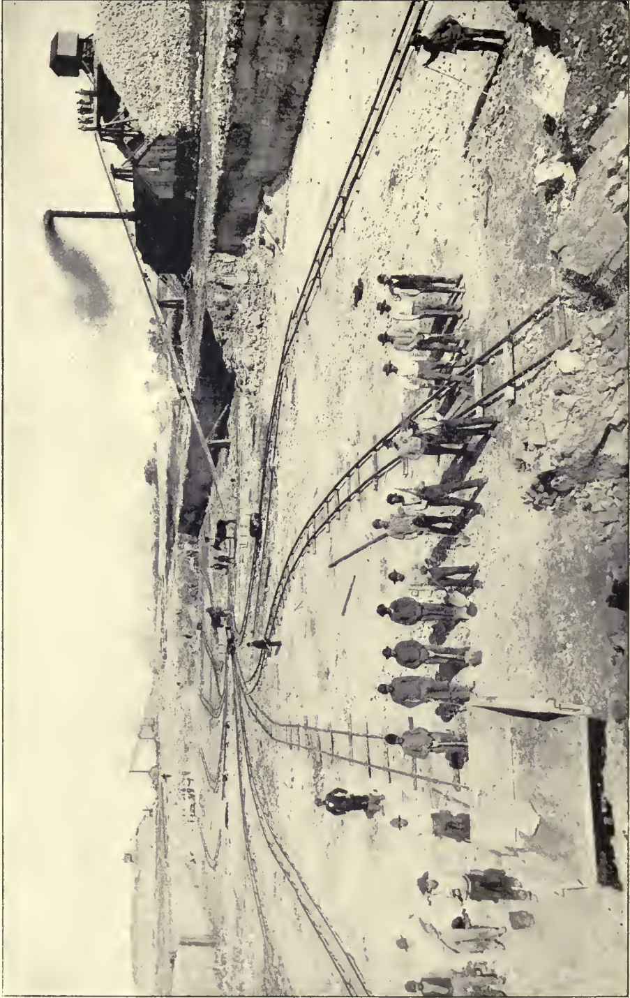
DRAINAGE CHANNEL AND WATERWAY IN ROCK. (FULL WIDTH AND ONE-THIRD REQUIRED DEPTH.)
