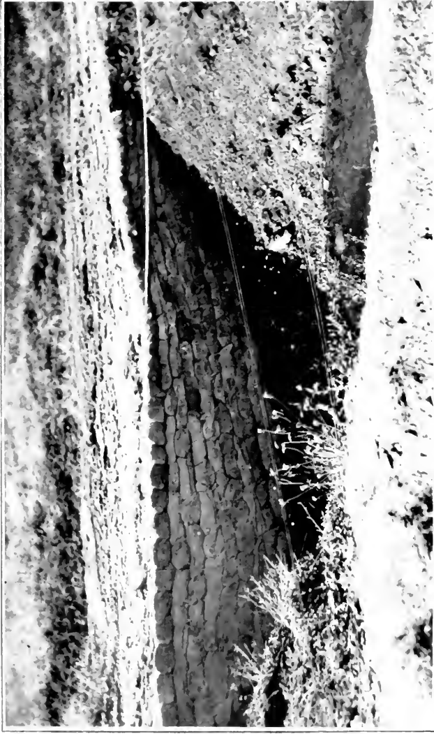
SAND BAG REVEMENT TO SUPPORT ROAD PASSING OVER PORTION OF A MINE CRATER.
