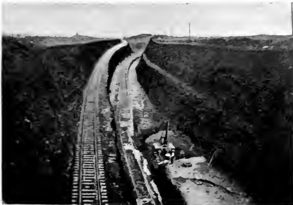
KIMBERLEY CUTTING WHEN IN COURSE OF CONSTRUCTION, SHOWING BOTH TEMPORARY AND PERMANENT LINES.
