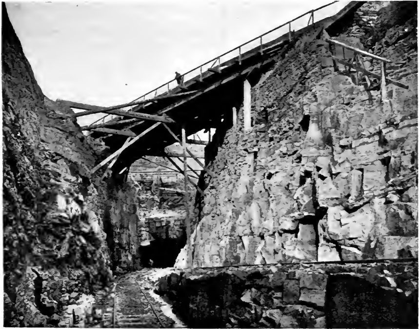
STRINES CUTTING AND QUEENSBURY TUNNEL, OVENDEN, NEAR HALIFAX, WHEN IN COURSE OF CONSTRUCTION.
