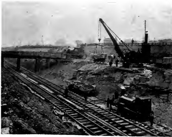
WIDENING THE LINE AT ARMLEY, NEAR LEEDS. Showing the removing of "spail" earth.
