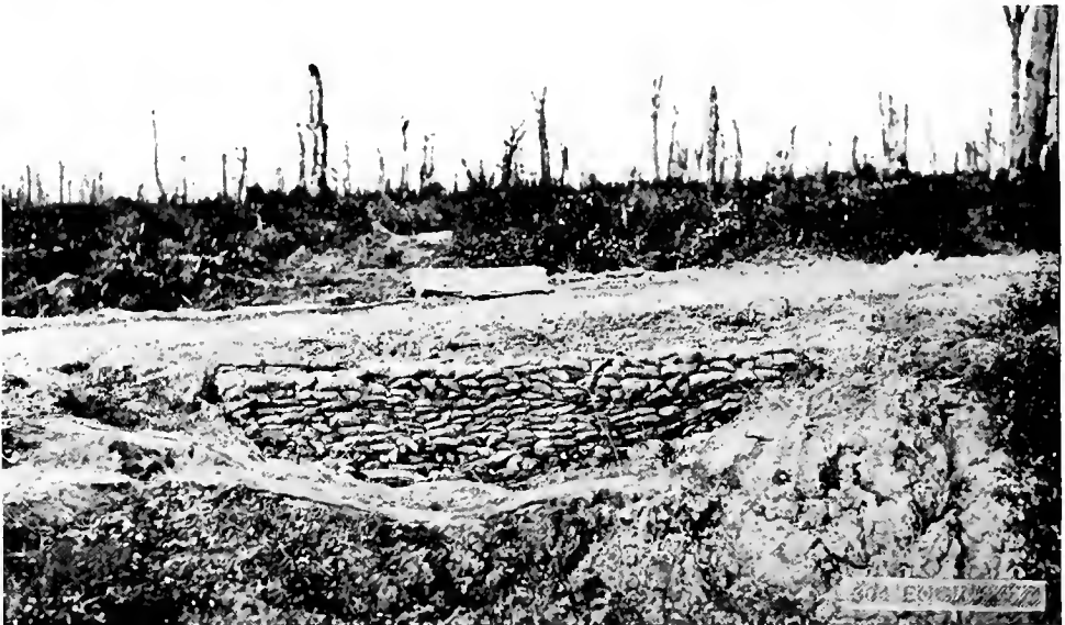
ROAD OVER NO-MAN'S LAND, RECONSTRUCTED BY 304 ENGRS., SHOWING METHOD OF FILLING SHELL HOLES.
