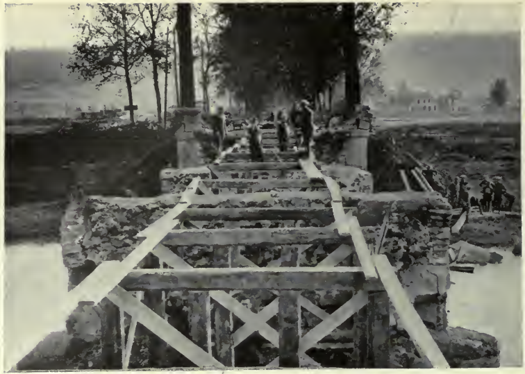
Under almost constant enemy fire, our 303rd Engineers repaired necessary bridges over the Aire River.
