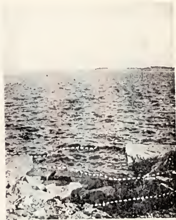
PORTION OF SEA WALL DAMAGED BY PREMATURE EXPLOSION.
