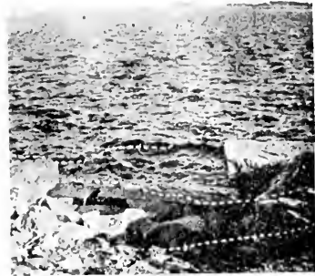
PORTION OF SEA WALL DAMAGED BY PREMATURE EXPLOSION.
