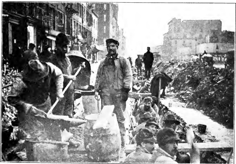
DETAILS OF LAYING TELEPHONE CABLES IN NEW YORK STREETS Bending Three-inch Iron Pipes for 38th Street Subway Rock Drillers in Trench
