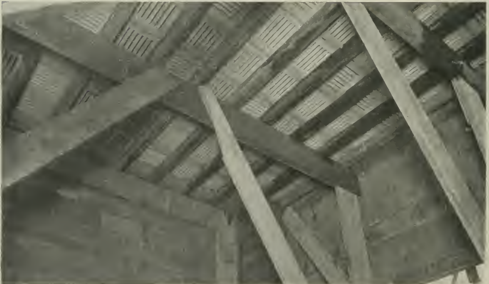
FIG 30. A TELLING ILLUSTRATION OF ECONOMY IN FORM WORK. THIS SHOWS THE UNDERSIDE OF THE SLOTTED PLASTER BLOCKS.
