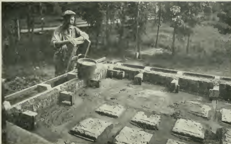
FIG. 16. THE FLUID CONCRETE IS Poured BETWEEN THE SAND MOULDS AND RISES AND FLOWS OVER THEM.
