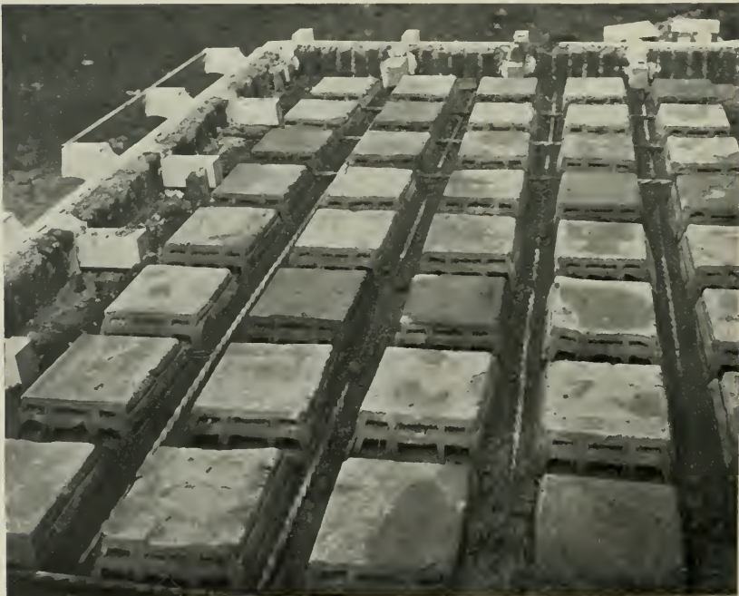
FIG. 25. THE CONTACT ALL ALONG THE BOTTOM MAKES EACH BLOCK IMMOVABLE AND PRESENTS AN ALL-TILE CEILING.
