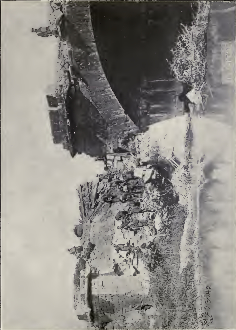
American engineers at work replacing a bridge across the Aire which had been dynamited by the Germans after retreating before the Franco-American assault.
