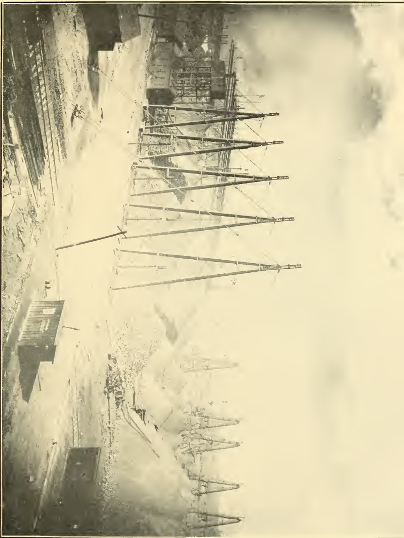
THE SECOND STAGE OF ORE UNLOADING. THE ORIGINAL BROWN PLANT ON THE N. Y. P. & O. DOCKS AT CLEVELAND UNLOADING BY CABLEWAY. THE FRONT TIER OF THESE MACHINES WAS MOVABLE. THEY WERE THE FIRST MOVABLE TIER CABLEWAYS EVER BUILT
