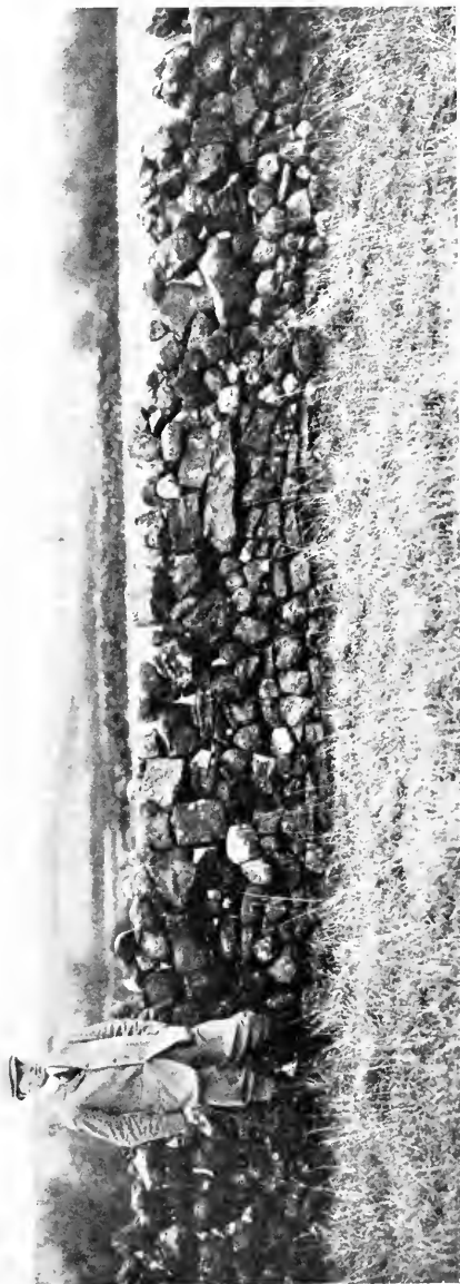
Fig. 119. — Loose stone wall.
