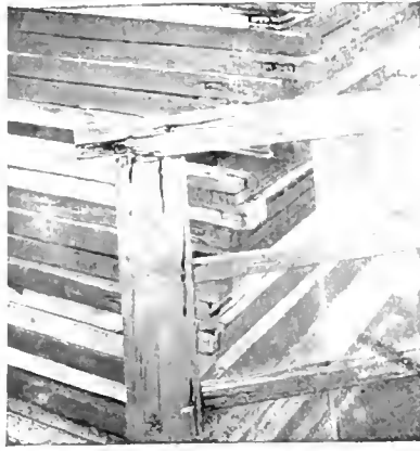
With the open mortise joint the water easily soaks in, and not only the side but every part of the joint decays.
