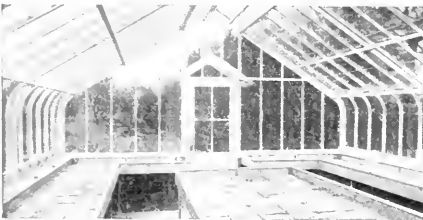
You know from the very look of it that it is the practical curved eave.
