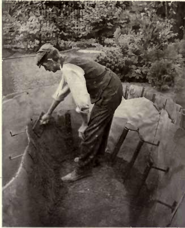
The site of the pool should be excavated to a depth of 2' or 3'. Concrete makes a good lining if a fairly rich mixture is used.
