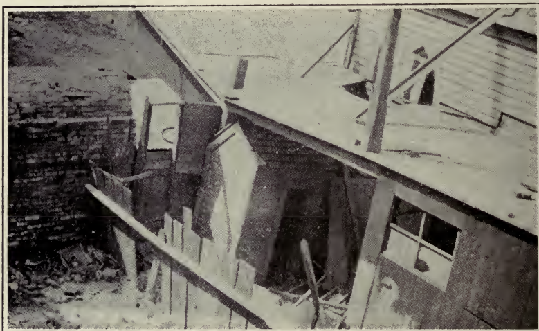
No. 33. Neglected vault, a source of yard pollution. Should be emptied and filled with clean earth.
