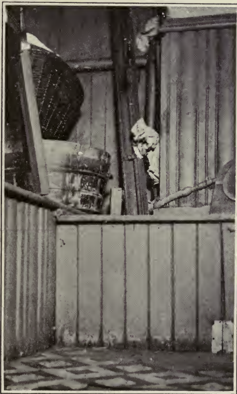
No. 32. Rotten enclosed plumbing as revealed by flashlight.
