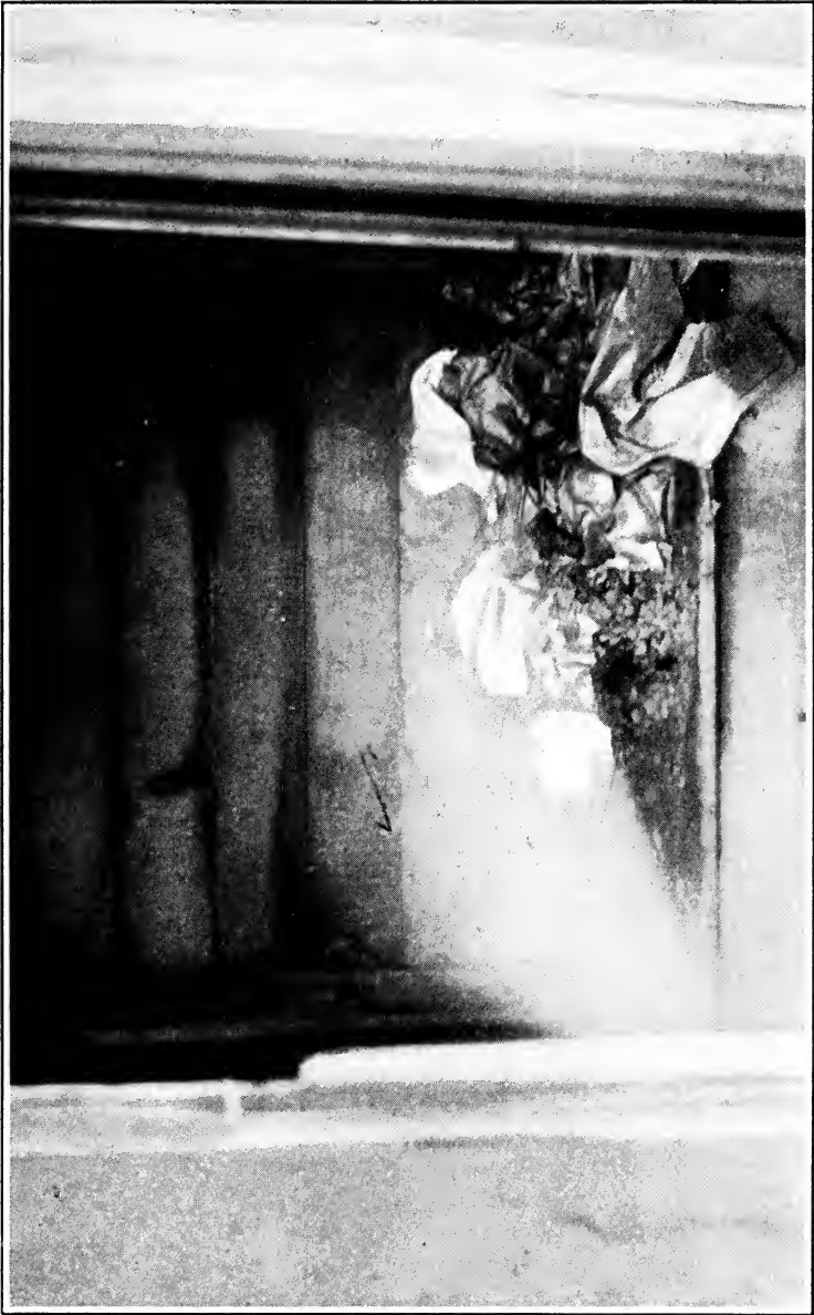
No. 30. An overflowing vault closet.
