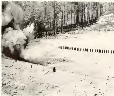
First blast for the stadium was made in late spring. To the right of flying debris, stumps mark the course of a drain under playing field. Work on the stadium lasted until fall.
