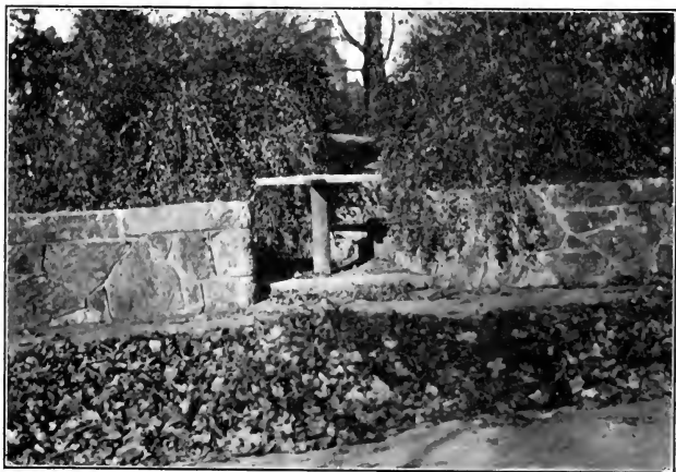
PLATE XIV. Well built wall, note raked out joints and slight batter. Turnstile instead of gate.
