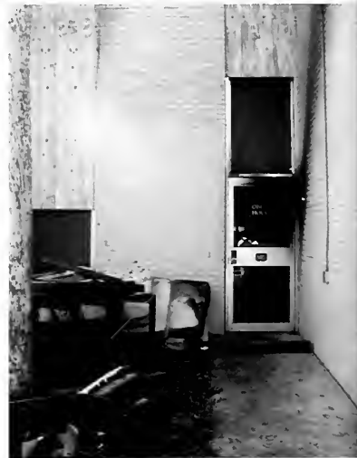
Repairs of Oberg after the fire left students without their rooms. The Oberg residents stayed at nearby facilities for the remainder of the school year while workers strived to repair the damaged house. photo by Joe Morris
