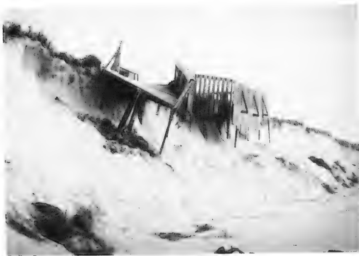
Photo 6. Damaged boardwalk, St. Joseph Peninsula State Park, Fla.
