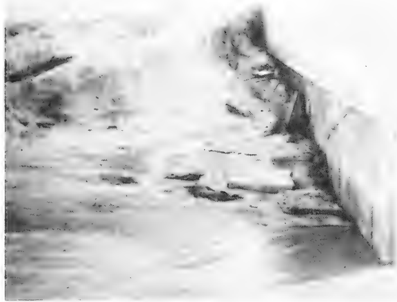
Photo 1. Erosion around end of seawall, Panama City Beach, Fla.
