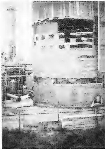
Photo 4. Damaged tank covering, Port St. Joe, Fla.
