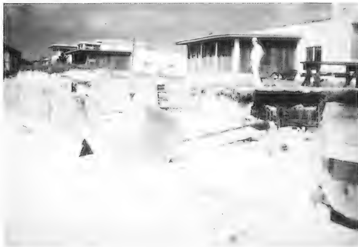
Photo 2. Destroyed seawall, Mexico Beach, Fla.
