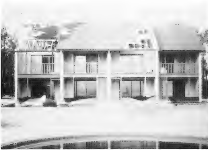
Photo 9. Roof damage, Cape San Blas, Fla.
