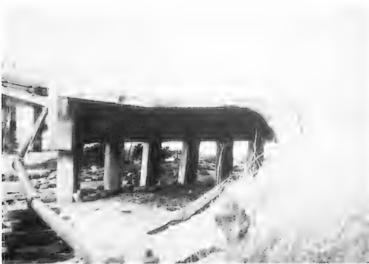
Photo 10. Highway damage, St. George Island Bridge, Fla.
