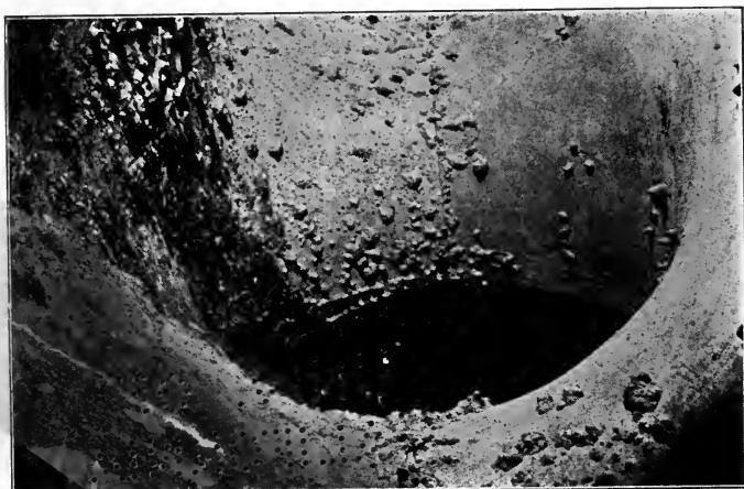
Tubercles Growing in Iron Water-pipes. Courtesy of Prof Gardner S. Williams.
