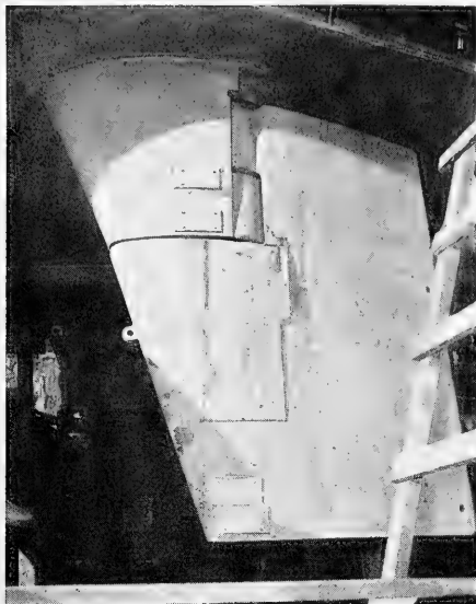
FIG. 75.E ROUGHNESSES AND DISCONTINUITIES ON A RUDDER HORN AND RUDDER
