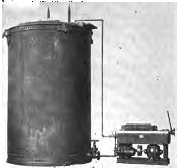
FIG. 283.—Method of Using Oil Dryer and Filter to Dry Oil in a Transformer as Installed.
