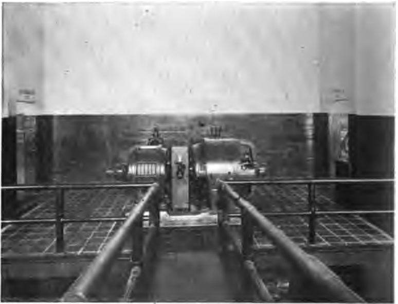
FIG. 215.—Exciter Set for Generating Unit in Mississippi River Power Company's Plant at Keokuk.
