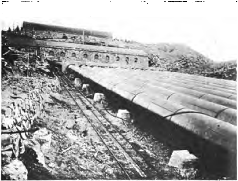
FIG. 60.—Ten Five-foot Riveted Steel Penstocks.
