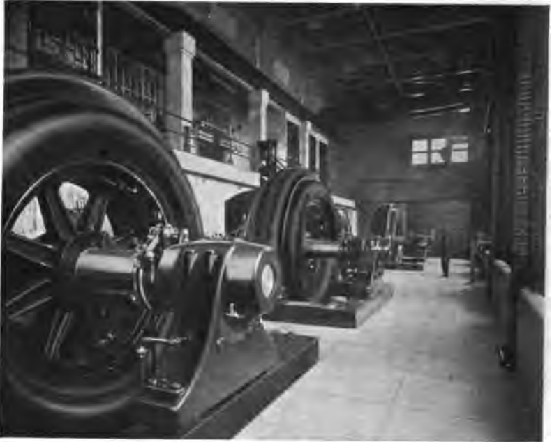
FIG. 91.—Interior View of Generating Station, Connecticut Power Company, Falls River Development.
