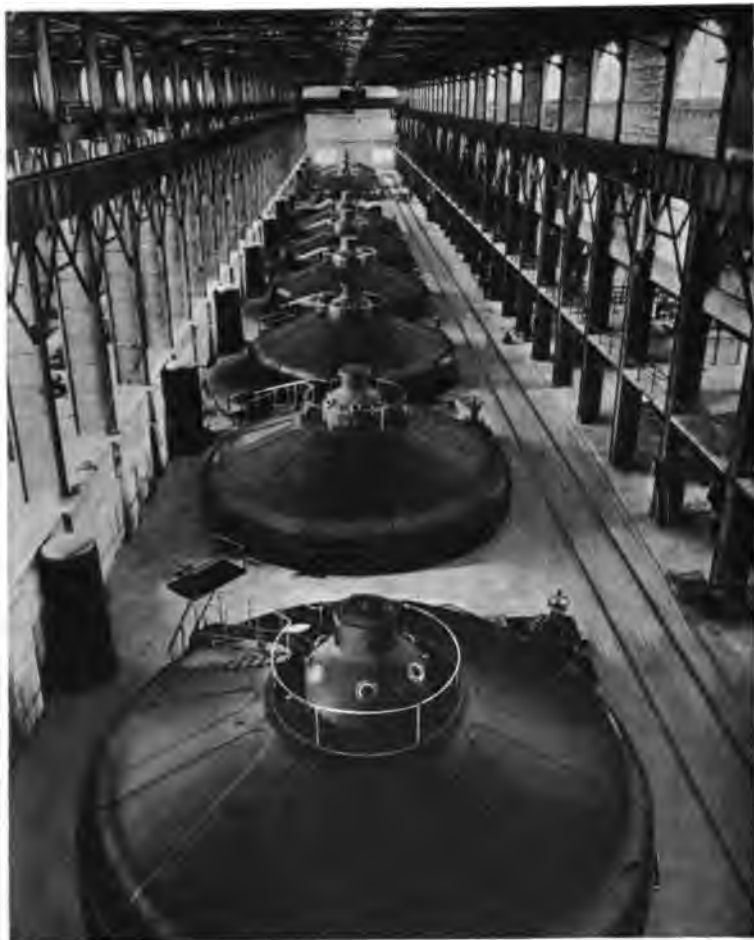
FIG. 90.—Interior of Generating Station, Cedar Rapids Mfg. and Power Company. Present Equipment, Ten 10,000 Kv.A. Generators. Ultimate Eighteen Similar Units.
