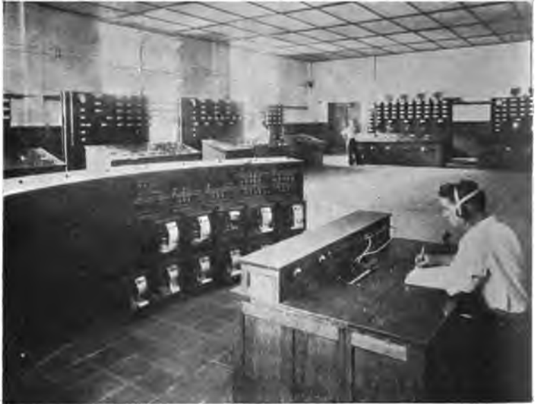
Fig. 344. —Mississippi River Power Company. Chief Operator's Room Showing Control Boards and Switchboards.
