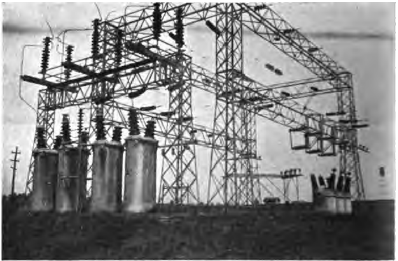
FIG. 389.—Outdoor Lightning Arrester Installation.
