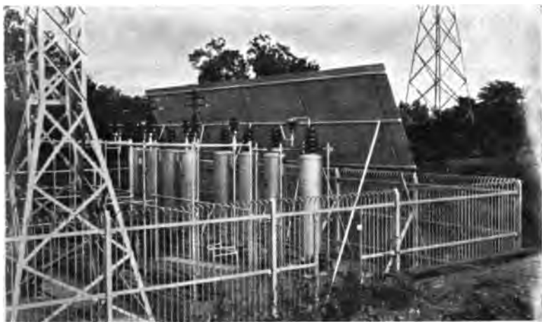
Fig. 390.—Outdoor Lightning Arrester Installation Showing Protecting Shield against Sun.
