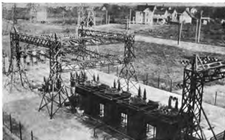
FIG. 369.—66,000-volt Outdoor Substation.
