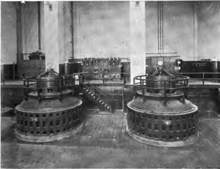
FIG. 216.—Auxiliary Generators with Direct-connected Exciters. Power Supply for Motor-driven Exciters shown in Fig. 215.
