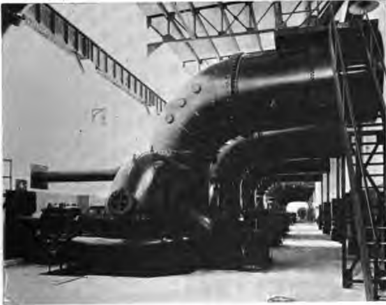
FIG. 120. —Double-runner Horizontal Turbines with Cast-iron Spiral Case and Double Discharge Tube. Hydraulic Power Company, Niagara Falls. (Built by I. P. Morris Company.)
