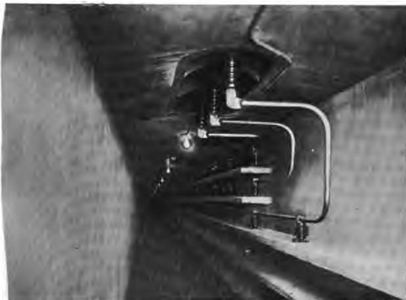
FIG. 371.—Showing Method of Bringing Low-tension Leads from Outdoor Transformers to Building through a Tunnel.
