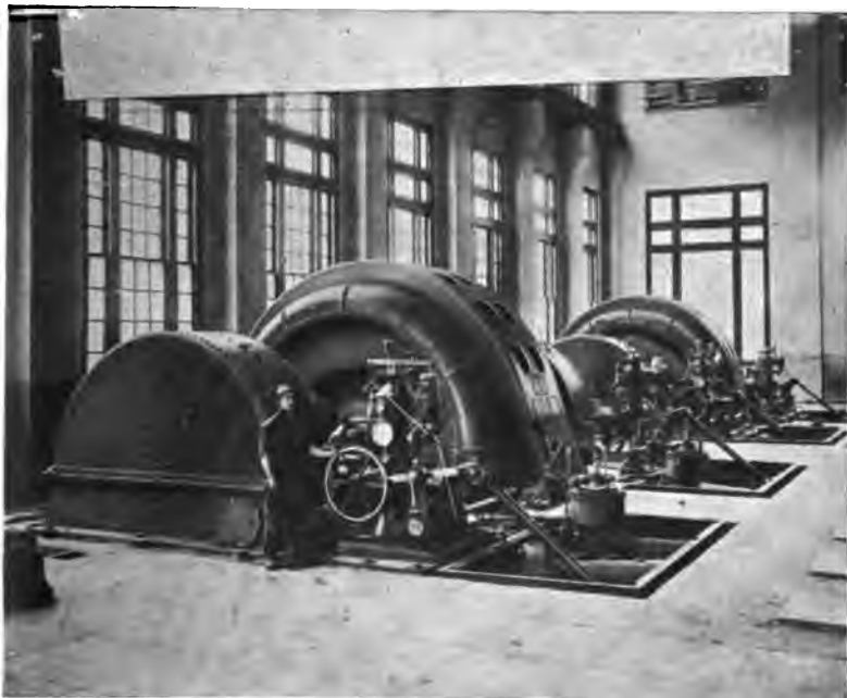
FIG. 92.—Interior View, Big Creek Development, Pacific Light and Power Company. 17,500 Kv.A. Generators.
