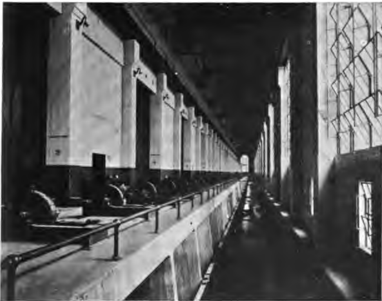
FIG. 75.—Gatehouse, Showing Gate-Lowering Mechanism. Mississippi River Power Company.
