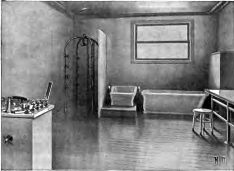
Fig. 80.—Interior hydriatic room at the Medical Bath, 1709 Rittenhouse Street, Philadelphia, Pa. Showing douche table, uprights for circular and rain douche, full tub, and sitz-bath (J. L. Mott Iron Works).
