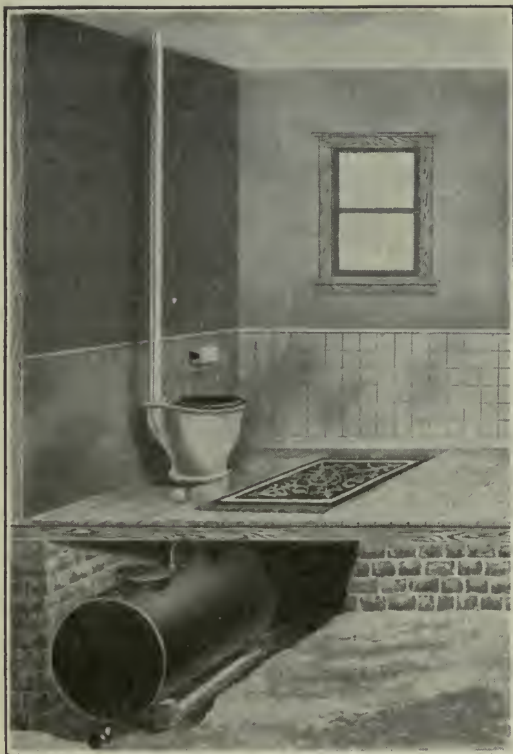
Fig. 38.—A Chemical Closet installed in a home where running water is not available. (Courtesy of The Dail Steel Products Company, Lansing, Mich.)
