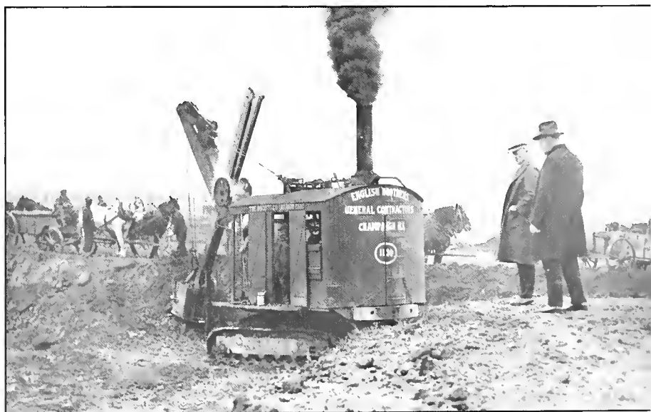
(L to R) Bob Zuppke and George Huff inspect digging for the foundation of Memorial Stadium.
