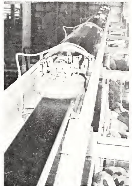
Feed drops onto a belt distributor in the confinement building. A brush take-off unit, oscillating between selected "stops," discharges feed into mangers beneath the distributor belt. Feed can be discharged to either side of the distributor belt. (Fig. 3)
