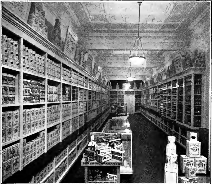
Fig. 8.—Semi-indirect gas fixtures as standardized for use in a chain of grocery stores.
