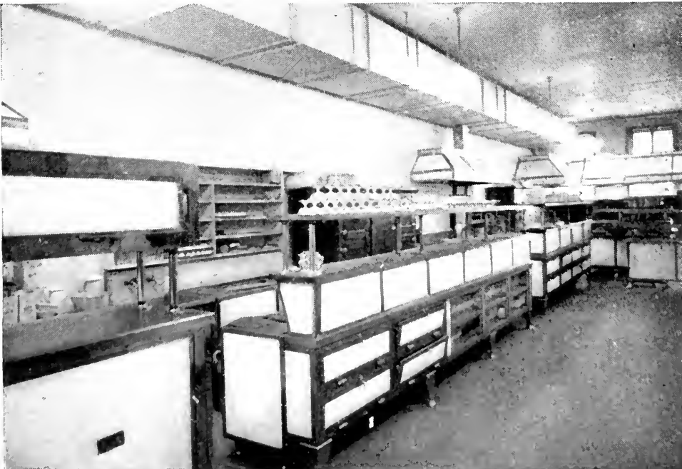
Fig. 24.—Typical restaurant kitchen using a luminaire of the enclosing glass type.
