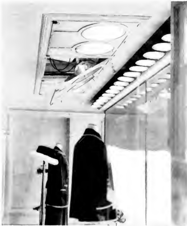
Fig. 2—Interior view of window showing equipment used. One of the frames is dropped to illustrate method of access for cleaning or lamp renewals.
