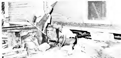
Plumbing Modernization at English Mansion without work since the closing of the Charlestown plants.
