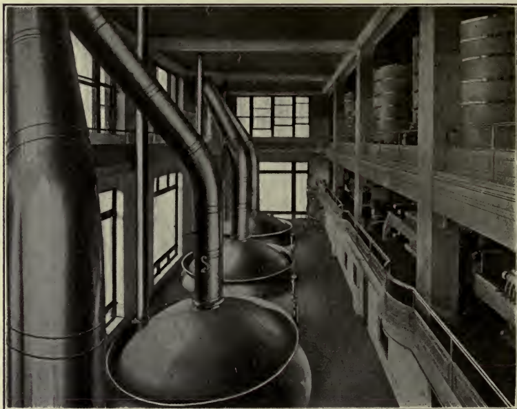
Fig. 46.—Copper Boilers. (Courtesy of United States Brewers' Association.)
