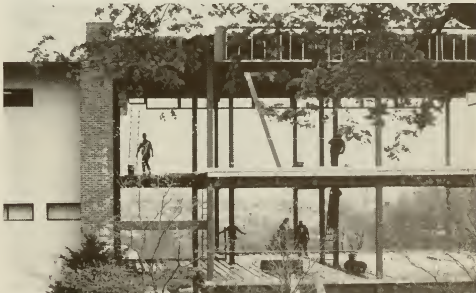
PROGRESS—Construction of the $1.7 million addition to the Jacob F. Buckman Hall of Engineering and Applied Science is well underway. Since the photo above was taken, workmen have encased the steel framework, bringing the project even closer to completion by September for the start of the academic 1990-91 year.
