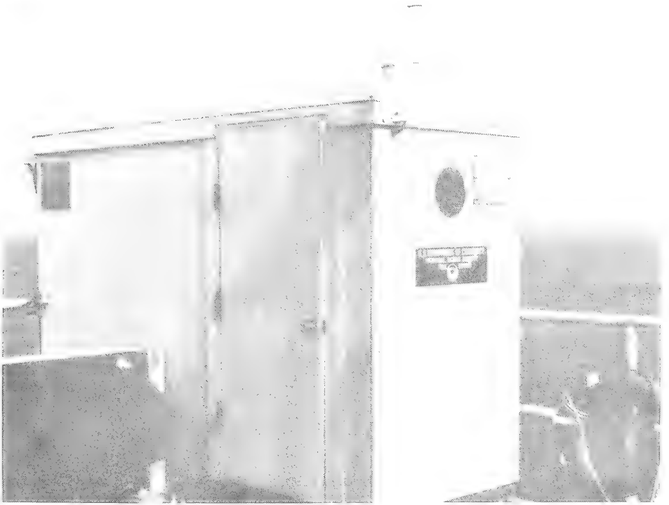
Figure 13. NOS control station at end of pier.
