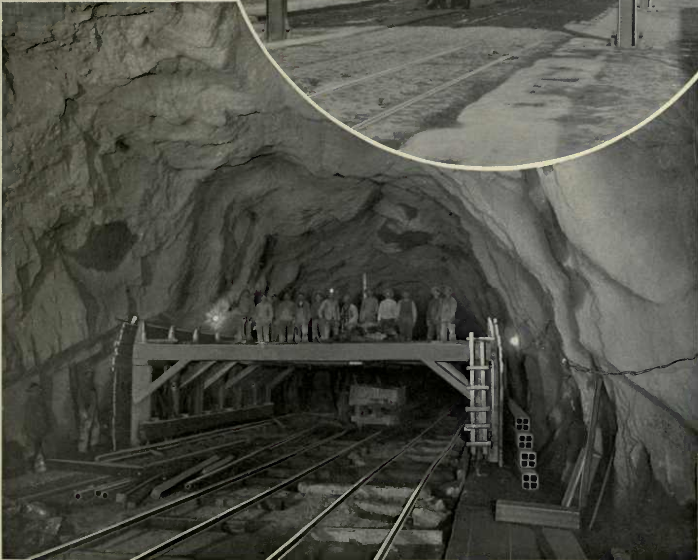
TRAVELER FOR ERECTING FORMS, CENTRAL PARK TUNNEL — (IN THIS TUNNEL DUCTS ARE BUILT IN THE SIDEWALLS)
