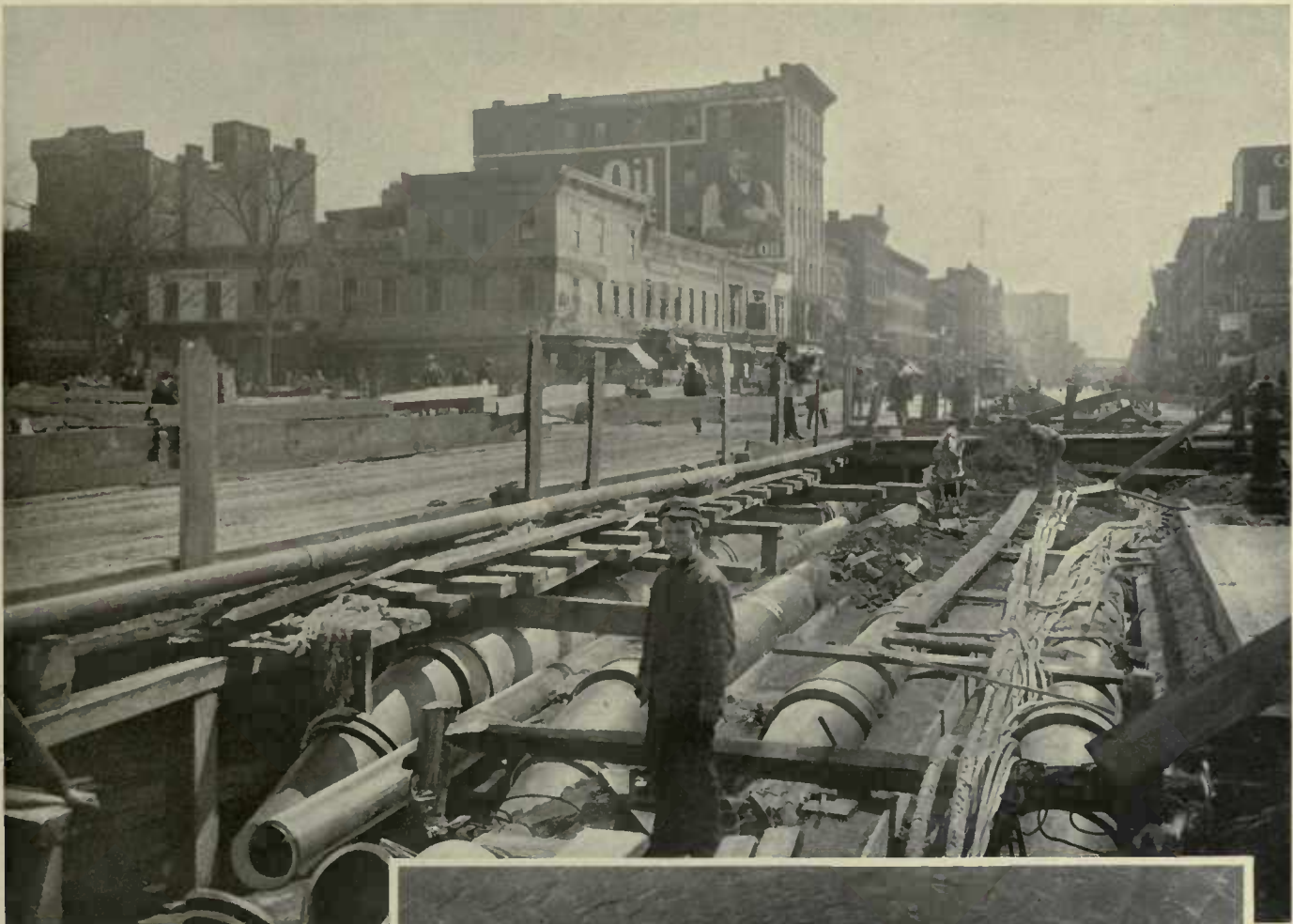
SMALL WATER MAINS BETWEEN STREET SURFACE AND SUBWAY ROOF, SUBSTITUTED FOR ONE LARGE MAIN — 125TH STREET AND LENOX AVE.
