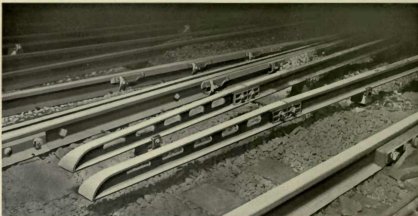
CONTACT RAILS, SHOWING END INCLINES
