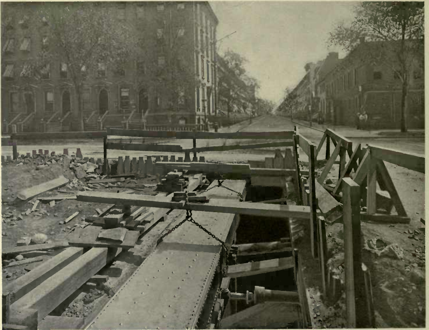
SPECIAL RIVETED RECTANGULAR WATER PIPE, OVER ROOF OF SUBWAY AT 126TH STREET AND LENOX AVENUE
