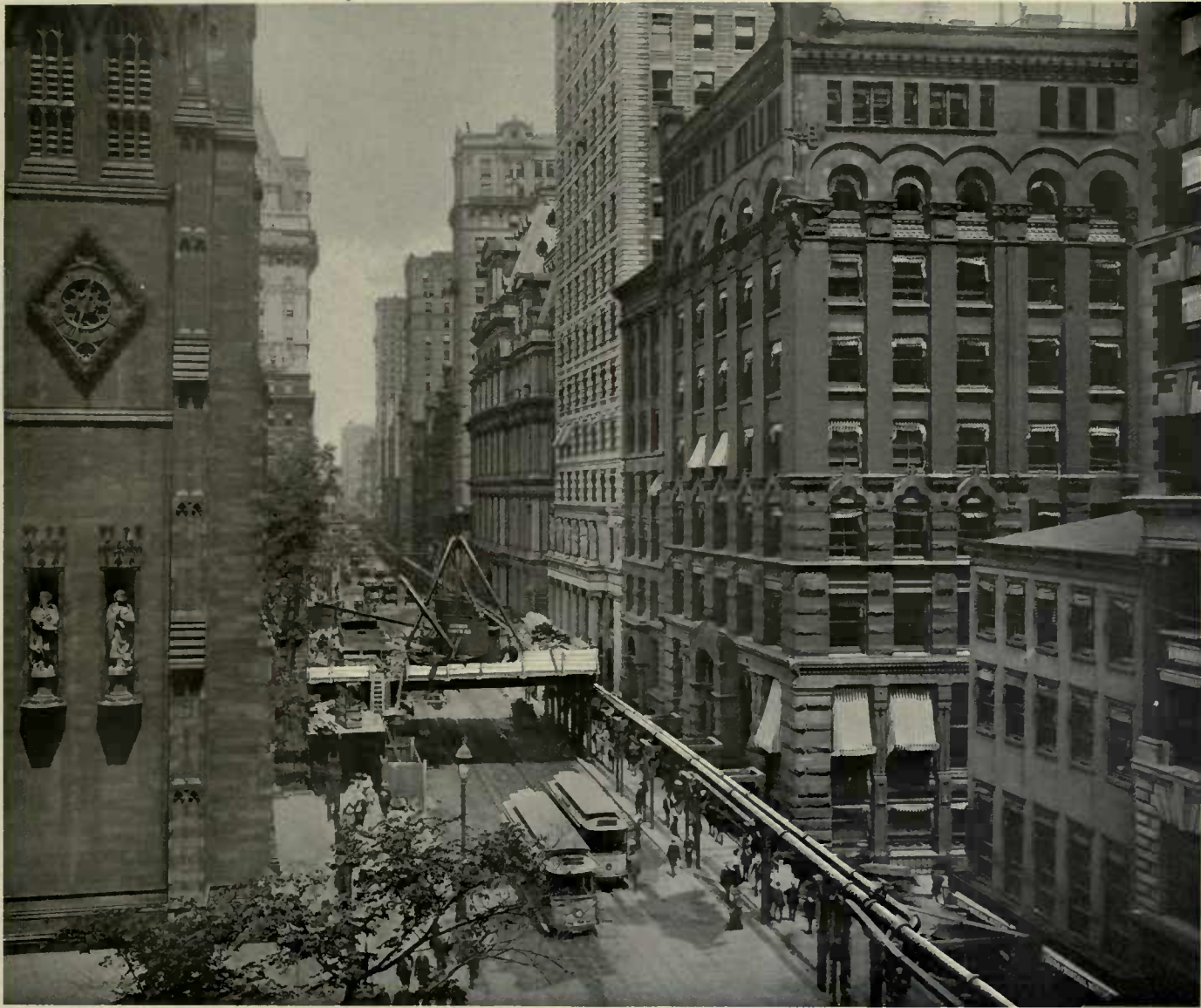
LOOKING UP BROADWAY FROM TRINITY CHURCH — SHOWING WORKING PLATFORM AND GAS MAINS TEMPORARILY SUPPORTED OVERHEAD
