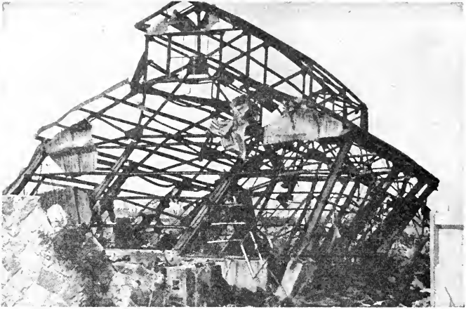
FIGURE 3.—Light, steel-frame industrial building, 1,800 feet from ground zero (ground point directly beneath the explosion). Corrugated iron roof and wall sheathing were stripped by the blast, and the combustible contents destroyed by fire.
