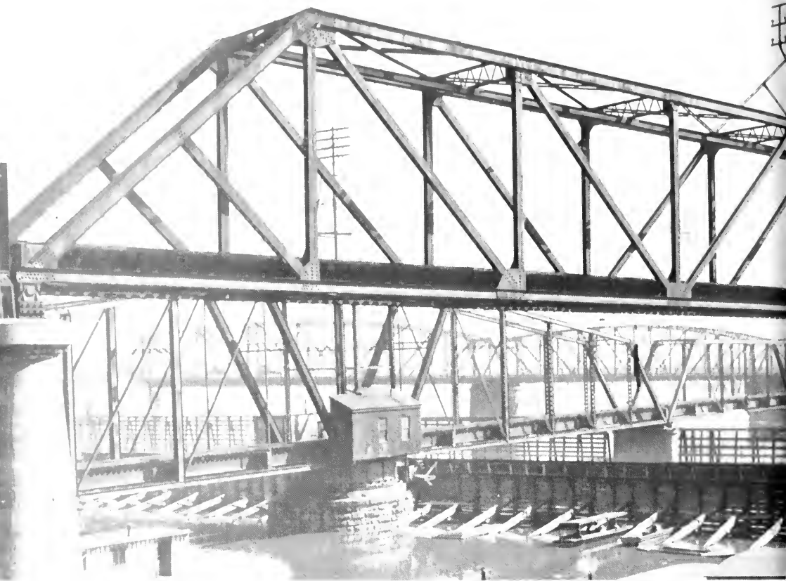
A typical Peoria-St. Louis limited train of 1925, made up of a handsome arch-roofed coach and matching parlor-buffet car with open observation platform, rolled across the jackknife draw span of Illinois Traction's substantial Illinois River bridge at Peoria. This structure became insignificant only in comparison with the company's Mississippi span at St. Louis. WILLIAM J. CLOUSER COLLECTION.
