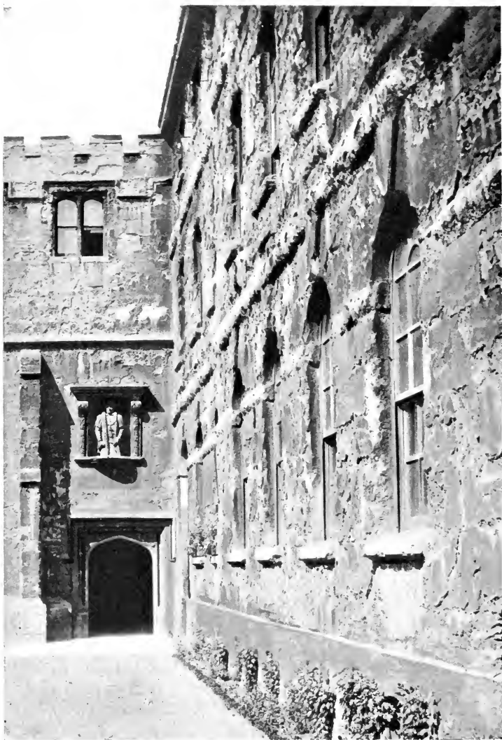
FIG. 57.—Weathering of limestone in the wall of an old building ; Trinity College, Oxford, England.
