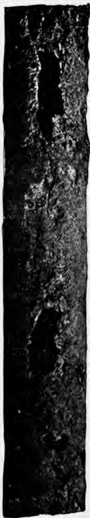
FIG. 29.—Wrought-iron pipe corroded in the soil.
