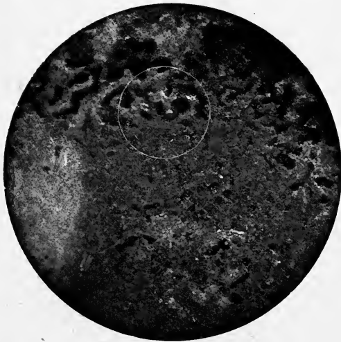
FIG. 39 (natural size).—Blisters, formed by warmth, in a red lead paint poor in varnish, topping a richer bottom coat. The blisters have burst, collapsed, and left the metal bare.
