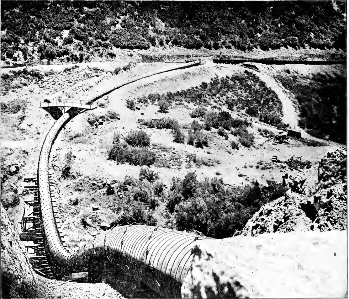
A WOODEN PIPE LINE OF THE BEAR VALLEY SYSTEM.
