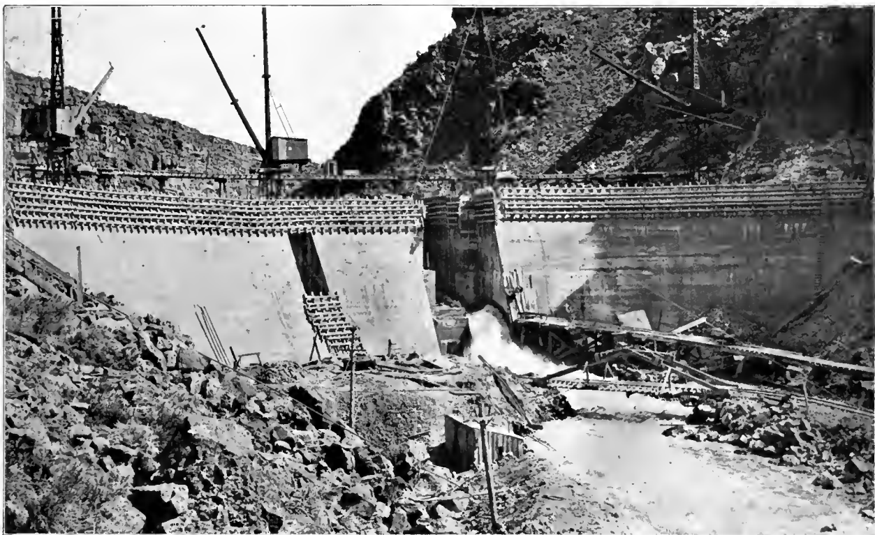
The Mammoth Salmon River Irrigation Dam, Twin Falls County, Idaho. A Close View of the dam when at a height of 80 feet looking south.
