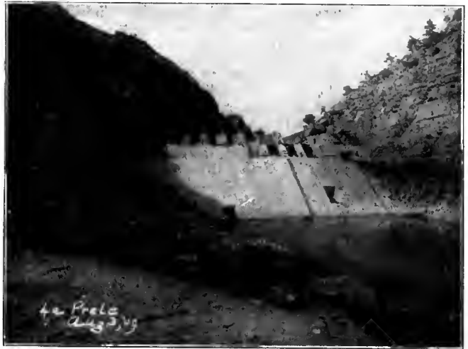
The Dam of the La Prele Irrigation Company, Near Douglas, Wyoming. It Is Now Completed and Is 135 Feet High. Will Store Enough Water for 25,000 Acres.
