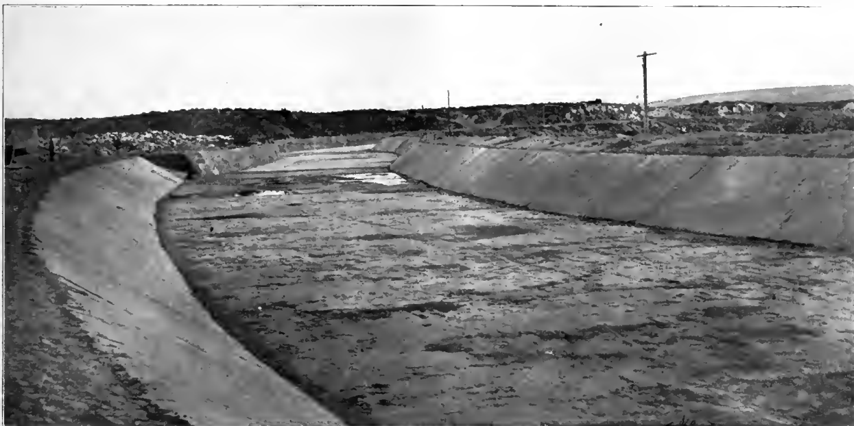
Main irrigation canal, Twin Falls North Side tract, showing treatment of canal banks through earth cut.
