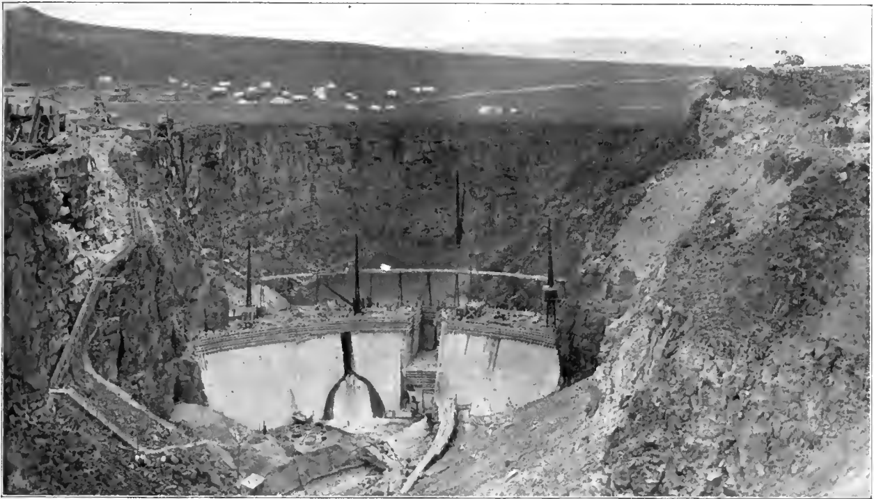
The Salmon River Irrigation Dam, Looking South from the Top of the Cliff. Also Showing Construction Camps.
