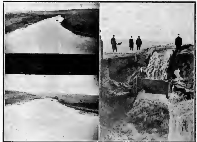
The two views on the left show Main Supply Canal; view on the right, Water Flowing into Reservoir No. 2, Fountain, Colorado.
