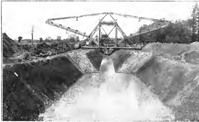
Ditch Being Dug with Sloping Banks—An Austin Drainage Excavator Ditch, showing variations in width made by same machine
