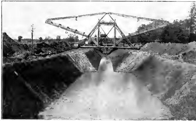
Ditch Being Dug with Sloping Banks—An Austin Drainage Excavator Ditch, showing variations in width made by same machine
