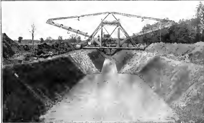
Ditch Being Dug with Sloping Banks—An Austin Drainage Excavator Ditch, showing variations in width made by same machine
