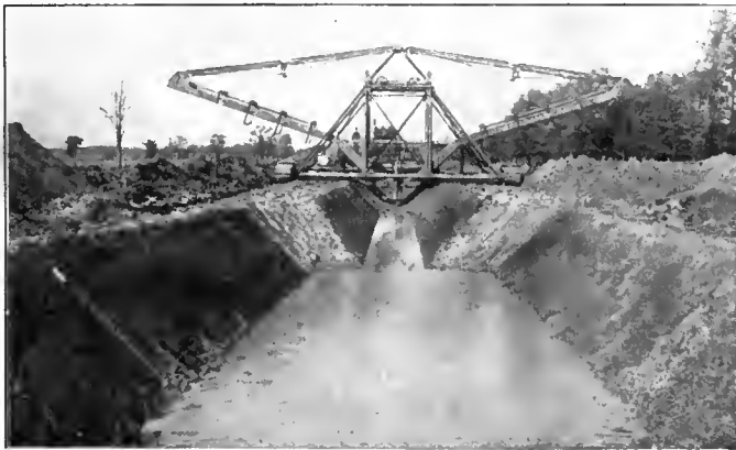
Ditch Being Dug with Sloping Banks—An Austin Drainage Excavator Ditch, showing variations in width made by same machine
