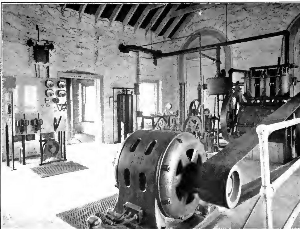
Interior of Main Power Station, Ryan Estate—The Gas Engine Is Operated by Producer Gas.
