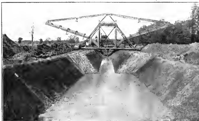
Ditch Being Dug with Sloping Banks—An Austin Drainage Excavator Ditch, showing variations in width made by same machine.
