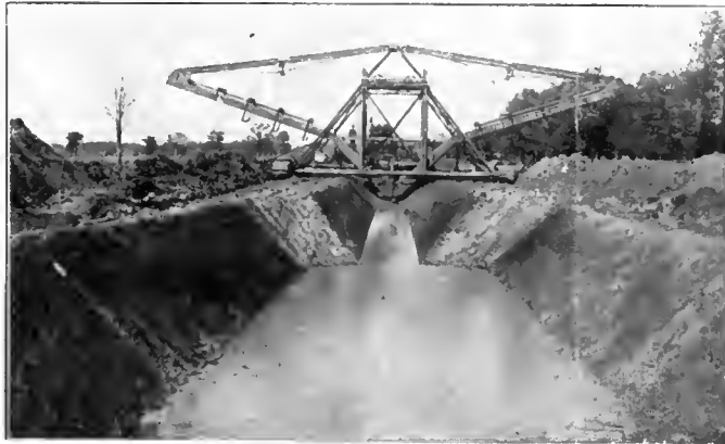
Ditch Being Dug with Sloping Banks—An Austin Drainage Excavator Ditch, showing variations in width made by same machine
