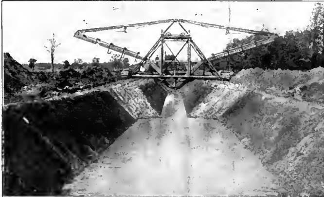
Ditch Being Dug with Sloping Banks—An Austin Drainage Excavator Ditch, showing variations in width made by same machine
