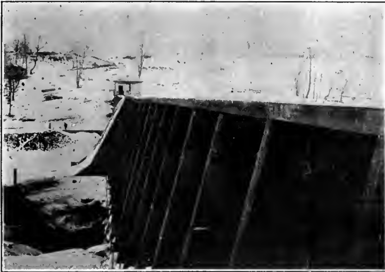
View of Blow-Out Showing the Slight Sag
